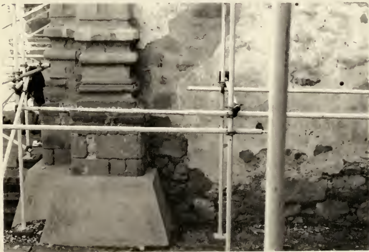
Fig. 15. North wall of east transept. Cementitious mortar repairs on stones, around edges of plaster, and as encasement of pilaster base at north wall of east transept.
